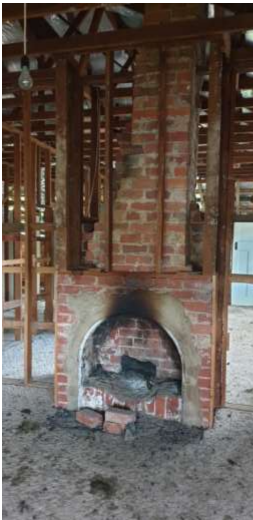
Figure 8 Double sided fireplace
